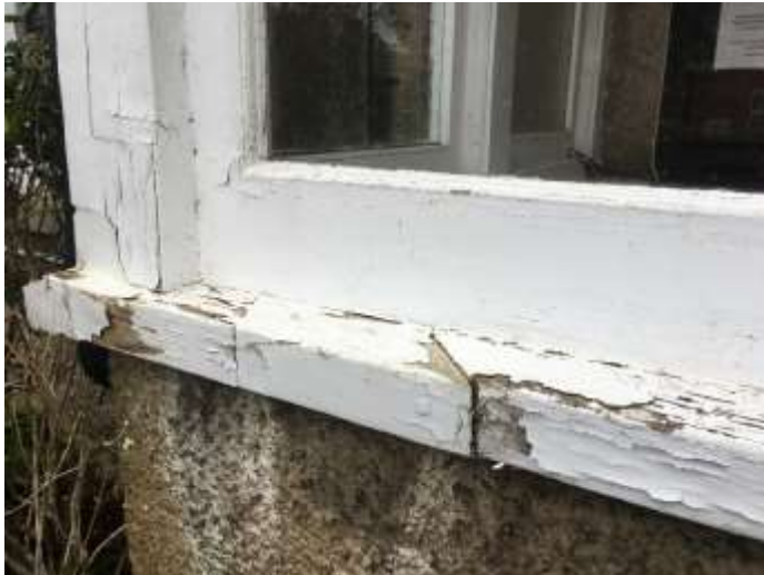
Photo 10 - The outside of the porch which has started to move
