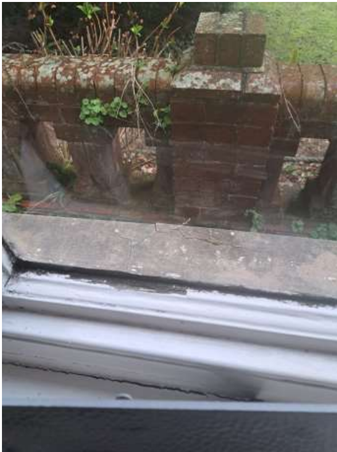
Photo 9 - more rotten windows
