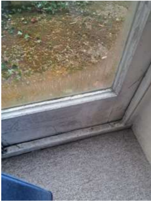
Photo 8 - another downstairs picture of mould and rotten doors.
