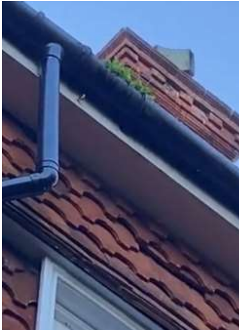
Photo 14 - The guttering is not maintained and as a result flooding and water ingress occurs.
