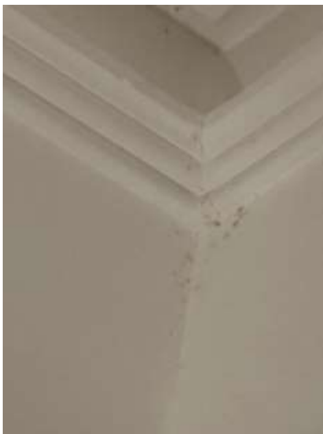
Photo 5 - mould on ceilings - this is one of the milder cases.
