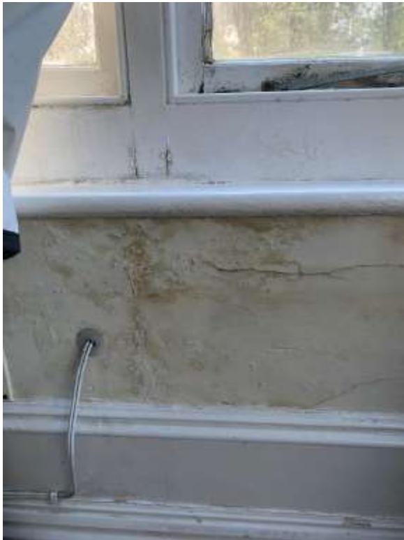
Photo 7 - Another downstairs flat. Drain pipes flooded due to lack of guttering cleaning and care.
