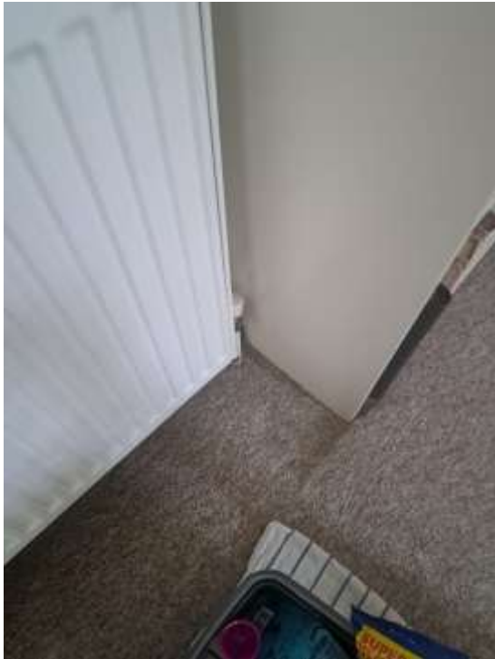
Photo 4 - Floor dipping by radiator, due to water ingress. Reported in 2018 - nothing has been done.
