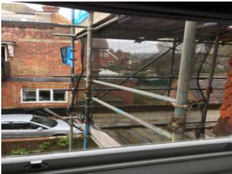
Photo 15 - I have had this scaffolding outside my window now for 18 months with no action nor repairs to the roof
