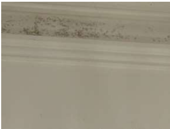
Photo 13 - More ceiling mould
